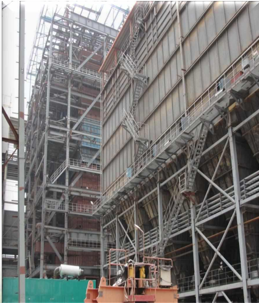
Unit 5 Boiler & ESP
