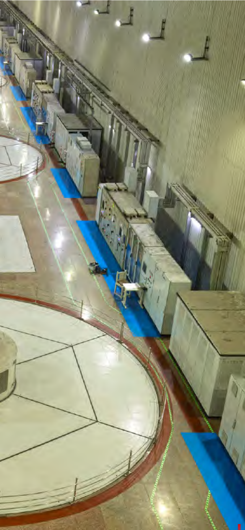
Turbine Floor, Baspa-II Power House
