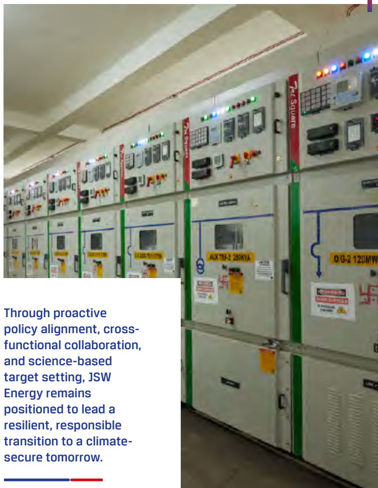
Electrical Panel Room
