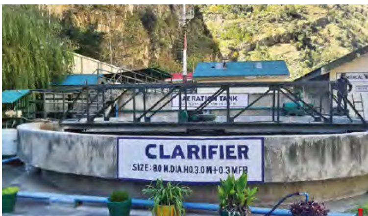
Water Treatment Plant, Sholtu
