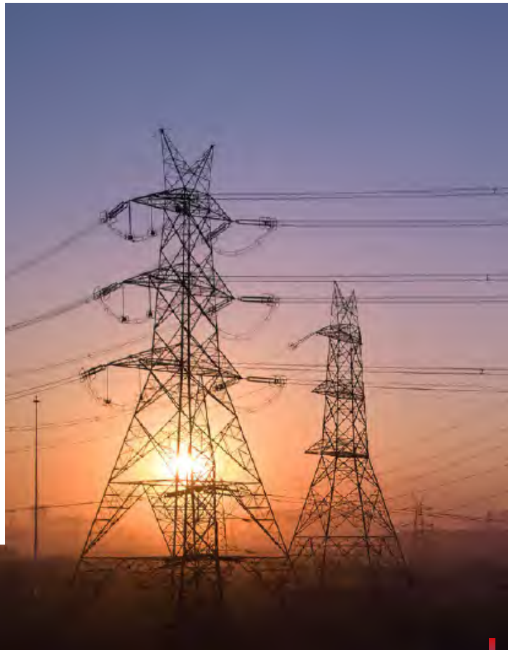
Power Transmission Line, Ratnagiri
