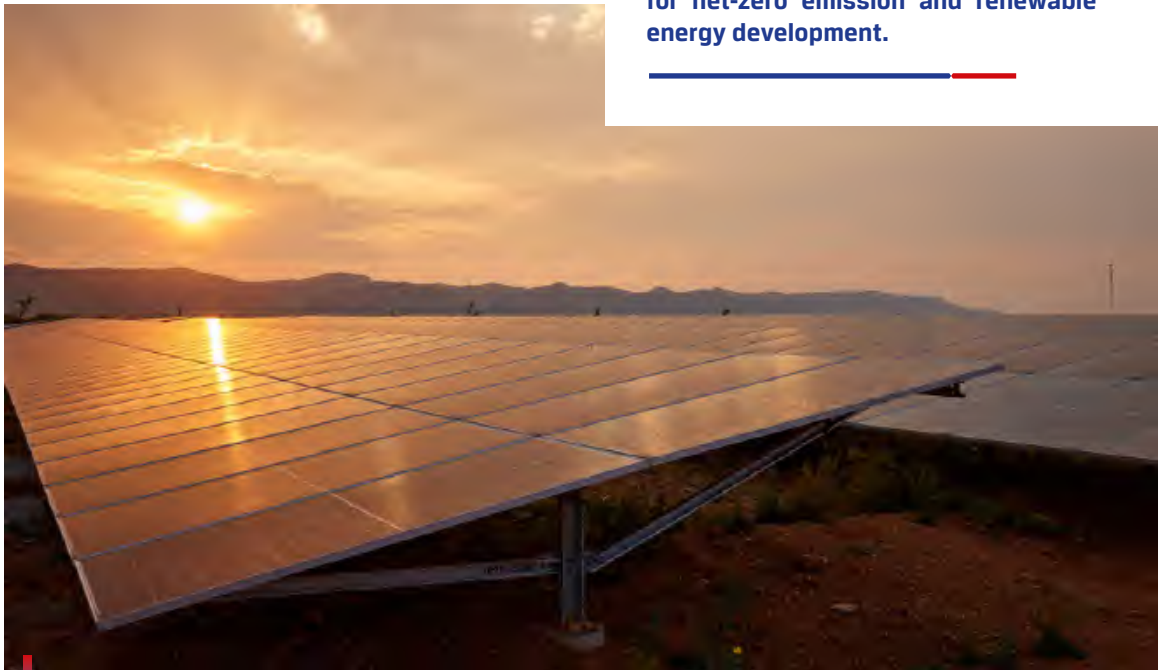
Solar Power Plant, Vijayanagar
