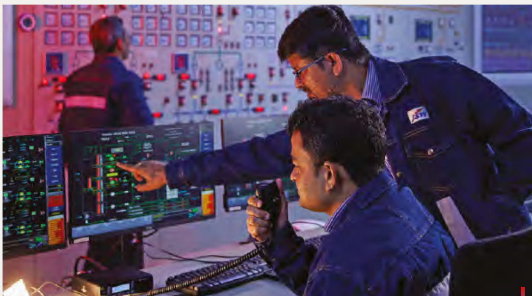
Thermal Power Plant, Vijayanagar
