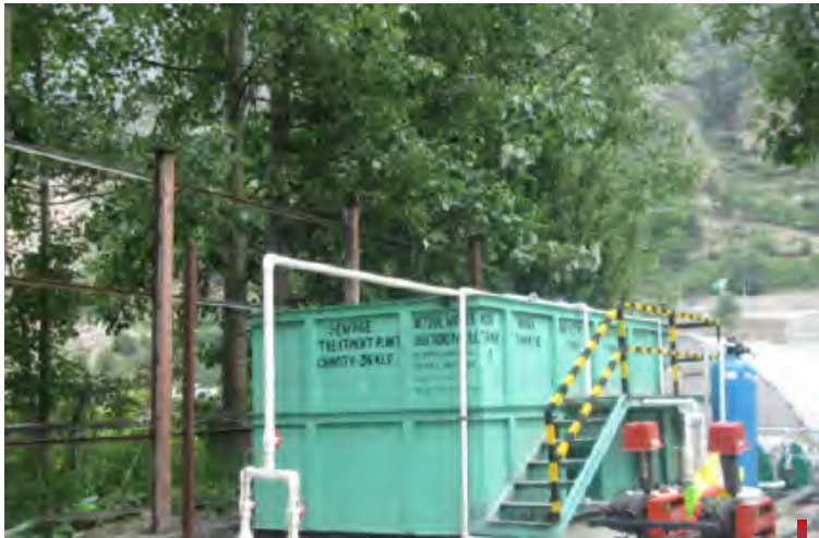
Sewage Treatment Plant at Sholtu
