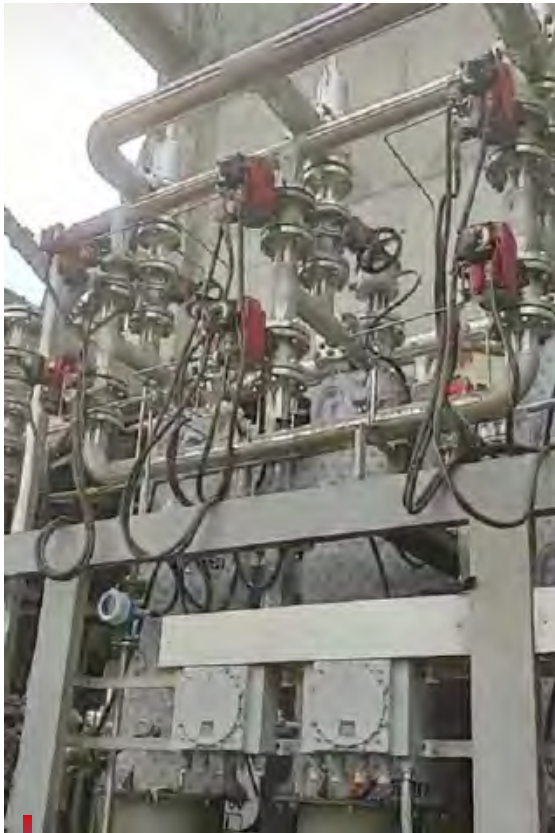
Green Hydrogen Plant, Vijayanagar
