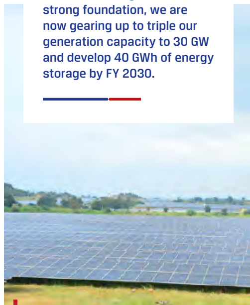
Solar Plant, Vijayanagar
