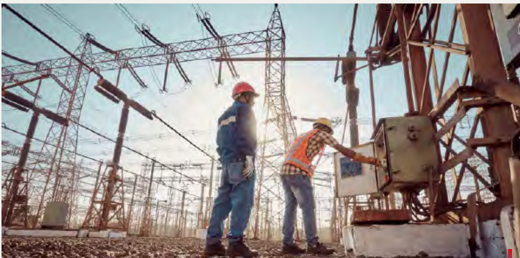
Switch yard, Vijayanagar Plant
