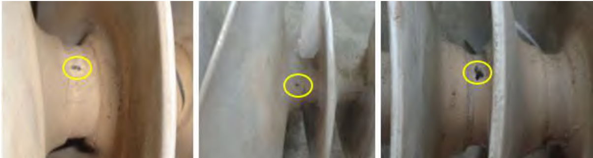
Figure 2.13: Punctures observed in different sections of SRI-2 insulator
