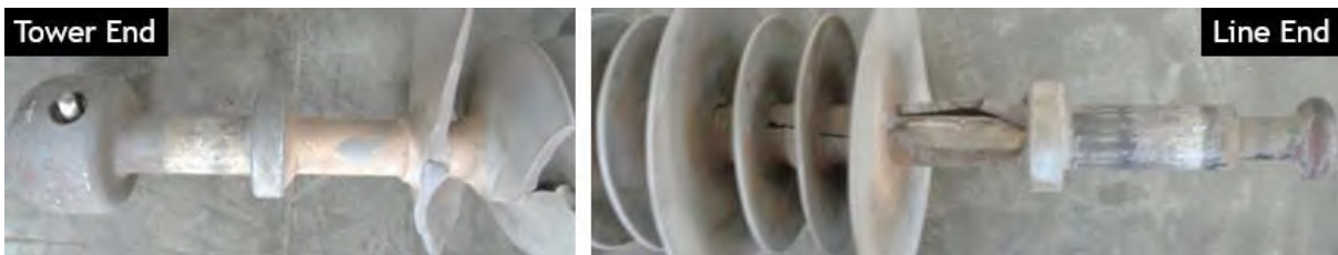
Figure 2.11: Both end of insulator the silicone shades are broken, silicone rubber seal at both ends are not directly affected
