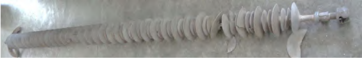
Figure 2.10: As received failed insulator (SRI-1) at the line end and tower end
