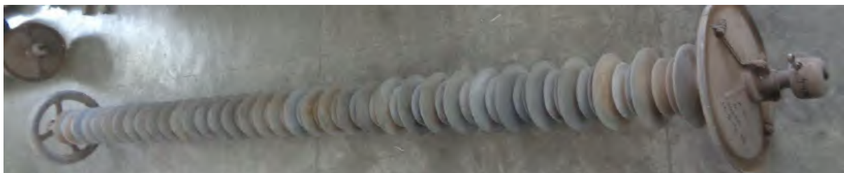
Figure 2.38: As received working insulator (SRI-6) received for analysis
