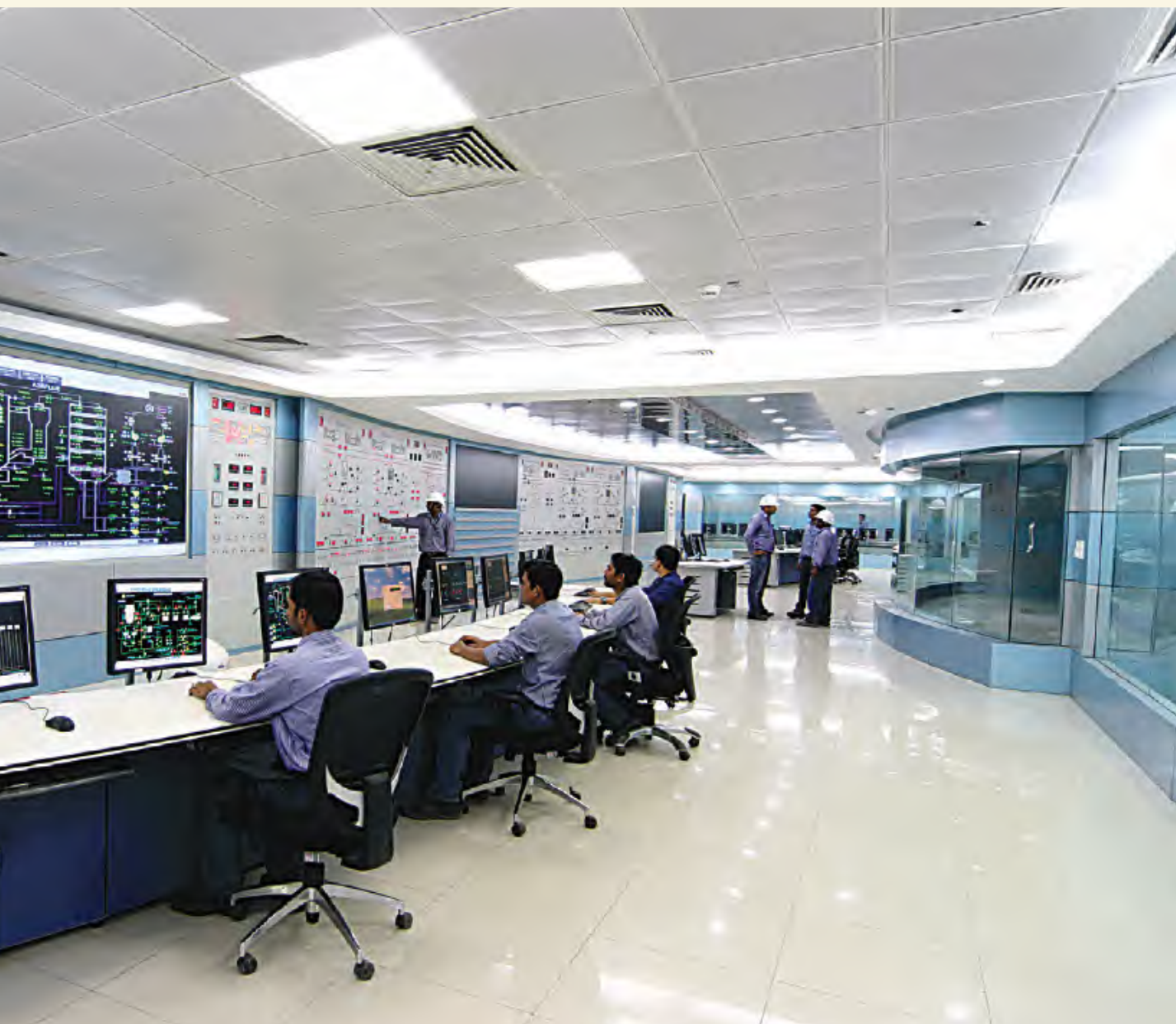
Control Room at the Vijayanagar power plant
