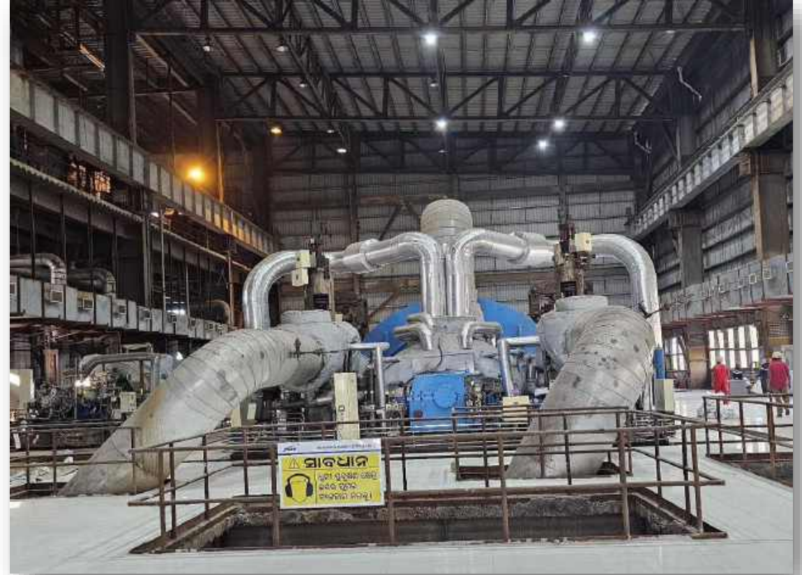
Unit 1 Turbine Generator set
