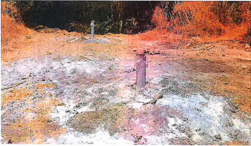
Figure 7. Two seepage monitoring well
