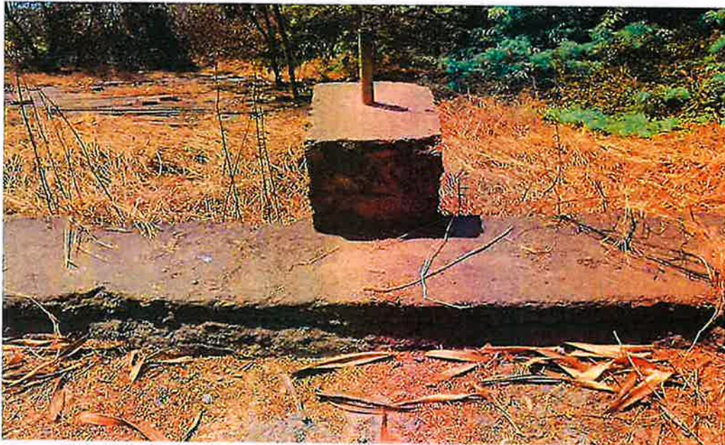
Figure 4. The sprinkler system stand pipe adjacent to the CC road
