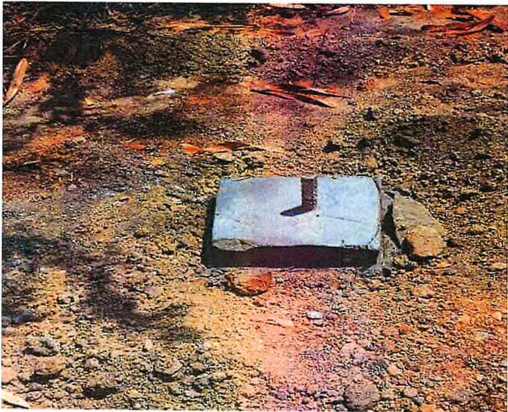
Figure 8. Settlement monitoring point
