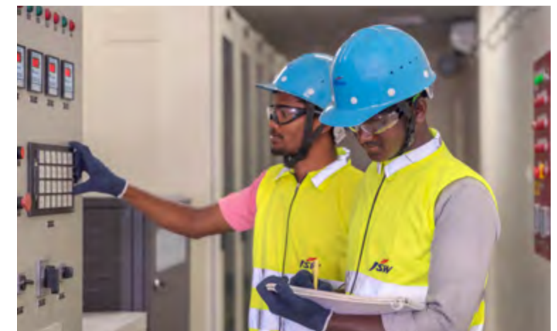
JSW Energy Tuticorin Wind power plant
