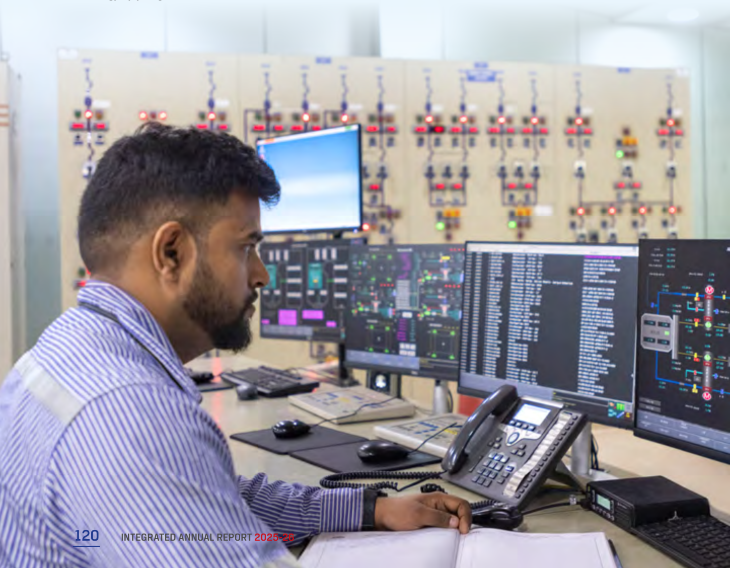
JSW Energy Vijayanagar Power Plant
