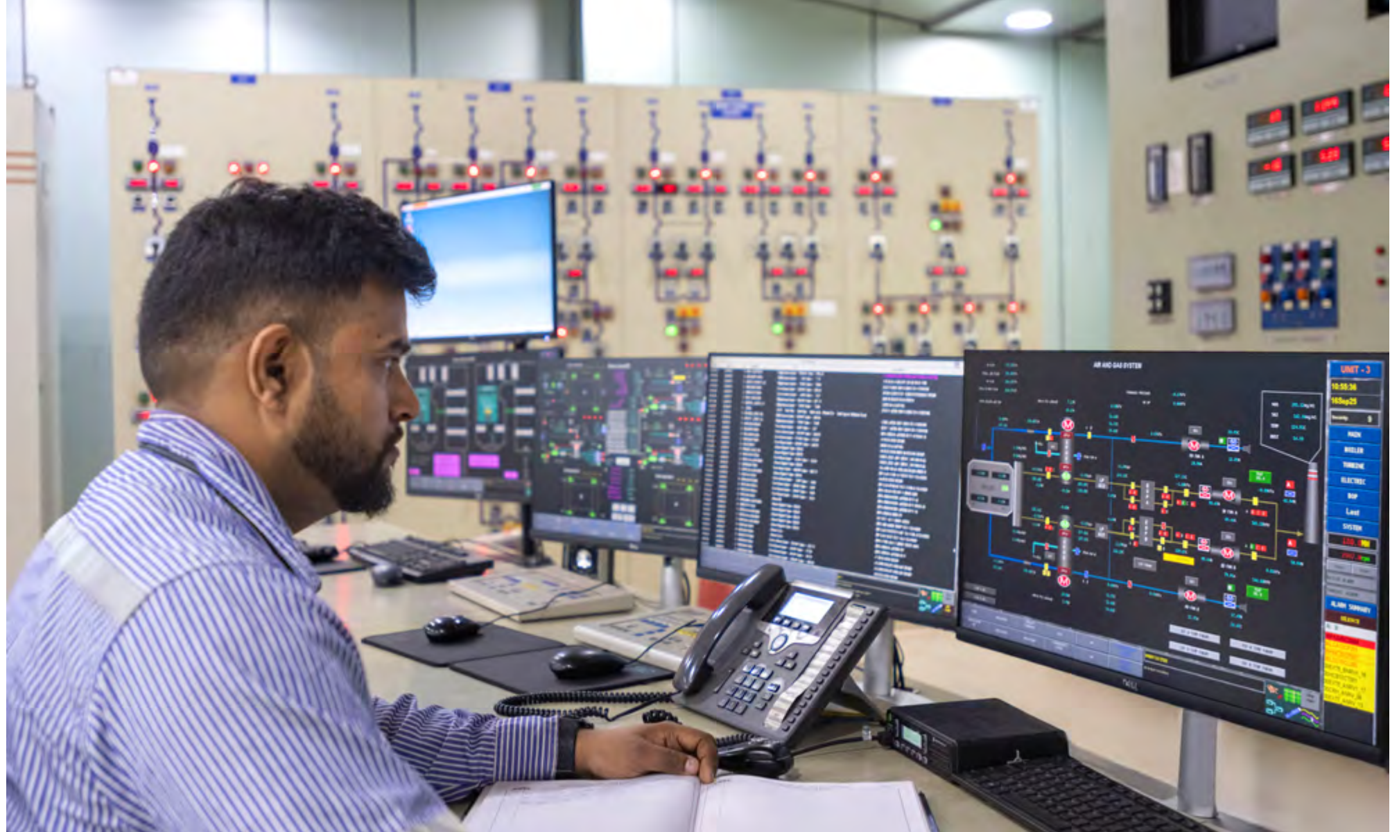
JSW Energy Vijayanagar Power Plant
