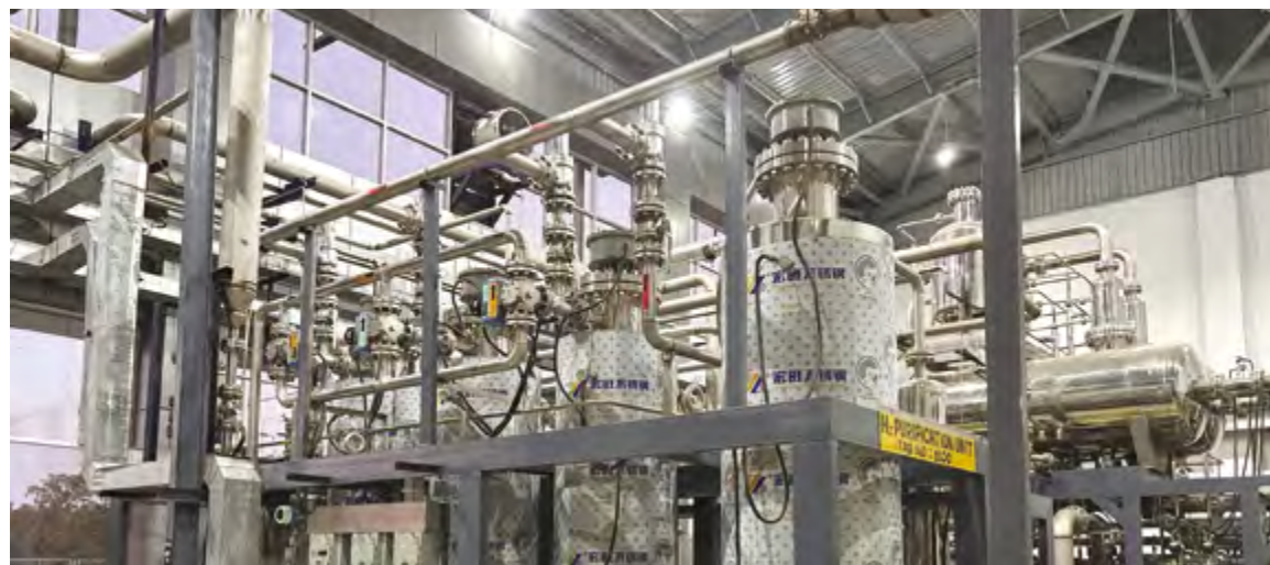
JSW Energy Green Hydrogen Power Plant
