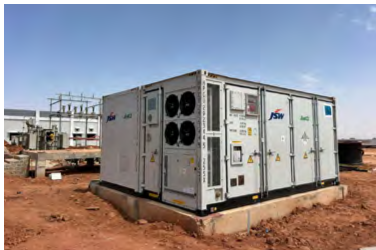
Battery Energy Storage Solution (BESS) Plant
