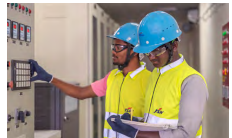
JSW Energy Tuticorin Wind power plant
