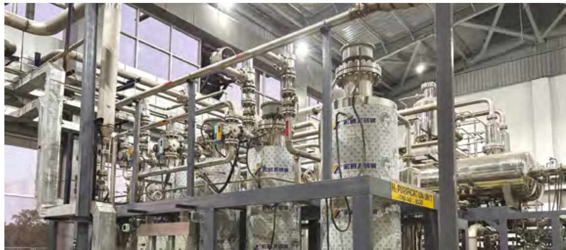
JSW Energy Green Hydrogen Power Plant
