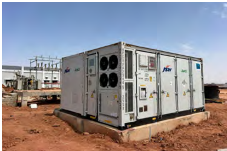
Battery Energy Storage Solution (BESS) Plant
