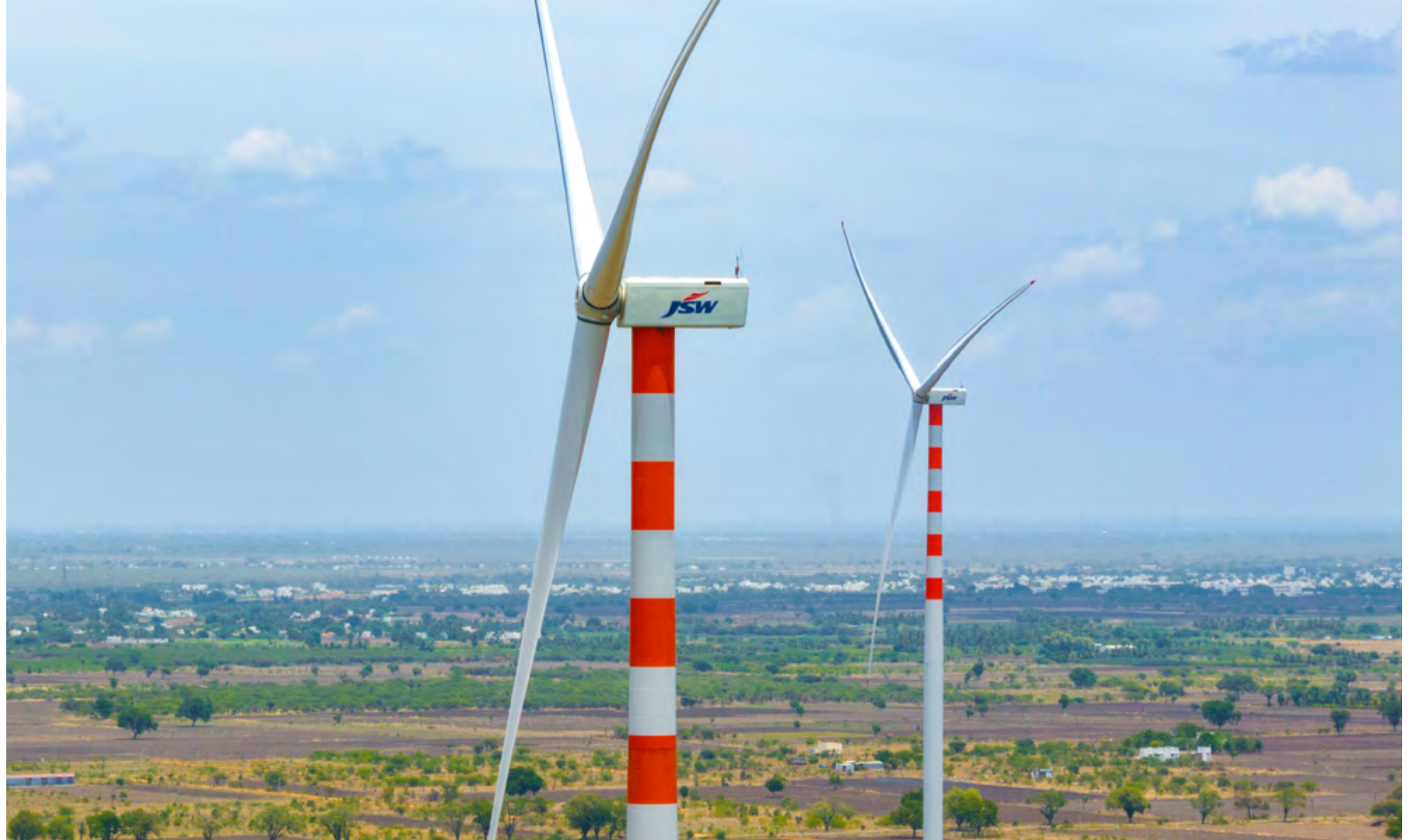
JSW Wind Energy Tuticorin Power Plant
